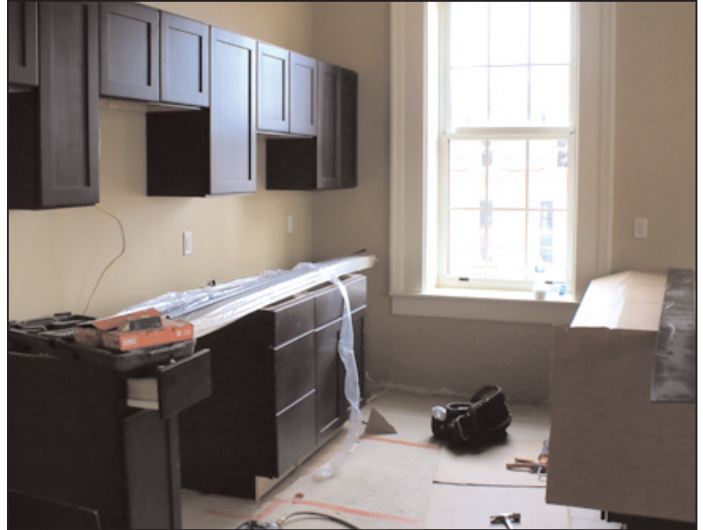
The Peabody Lofts will open around Sept. 1 and will consist of two bedroom, two full bathroom apartments with plenty of amenities. (Photo by John Hendler)
